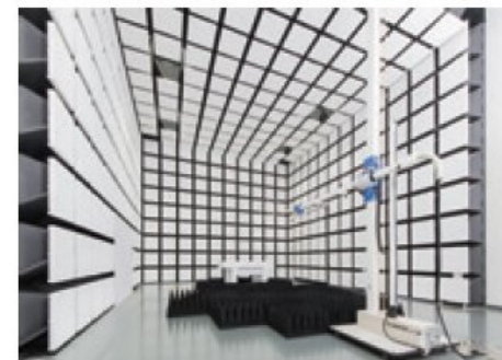
Electromagnetic shield room
